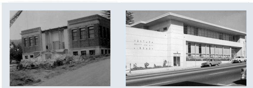
Here is the E.P. Foster Library building at the beginning of construction of the new addition in August 1958.
